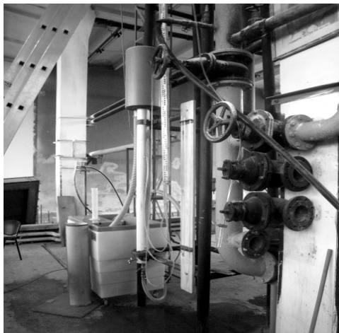
Photo 1. General view of the equipment with direct manometers
