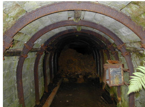
Fig. 1- The 3 ISEM collapse- gallery
