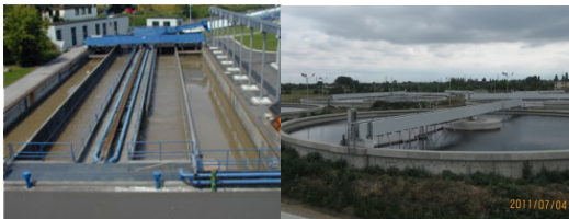
Fig. 4 Longitudinal and radial horizontal clarifiers. (source: http://www.aquatim.ro )
