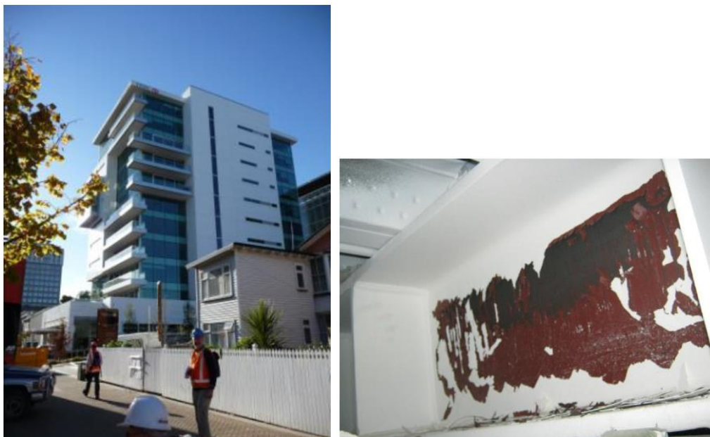
Fig. 2-40. Club Tower global view and paint peeling of EBF link [69]
