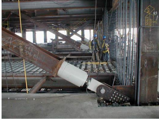
Fig. 2-6. Installed viscous fluid dampers on Torre Mayor Tower [10]
