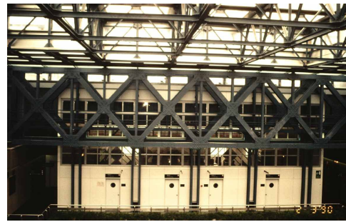
Figure 2-61 Trellis girders from the upper part of the Court in Ancona, Italy (Mazzolani) [159] by courtesy of F.M. Mazzolani
