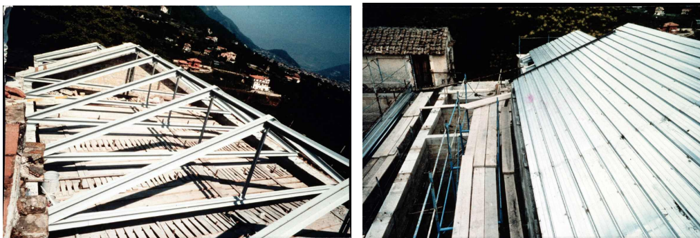
Figure 2-35 New steel roof structure of a restored church (Mazzolani) [159] by courtesy of F.M. Mazzolani
