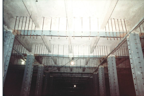
Figure 2-48 Consolidation of a reinforced concrete beam (Mazzolani) [159] by courtesy of F.M. Mazzolani
