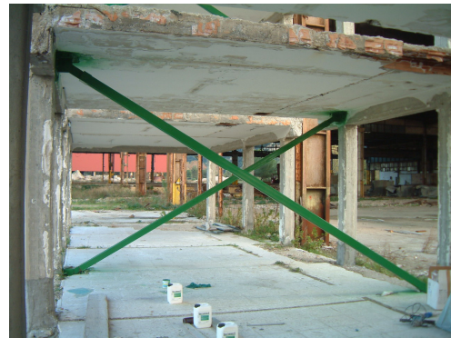
Figure 2-44 Reinforced concrete structure consolidated with BRB (Mazzolani) [159] by courtesy of F.M. Mazzolani
