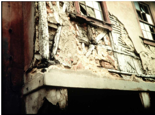
Figure 2-16. Damaged wooden structure(Mazzolani) [159] by courtesy of F.M. Mazzolani
