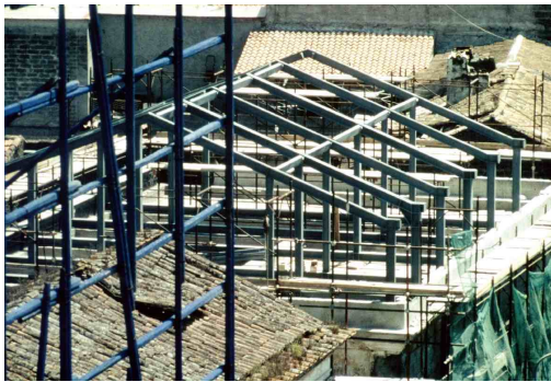
Figure 2-67 New roofing of Cultural Centre Succivo, Italia (Mazzolani) [159] by courtesy of F.M. Mazzolani
