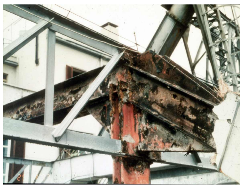
Figure 2-17 Corrosion phenomena in steel structure(Mazzolani) [159] by courtesy of F.M. Mazzolani
