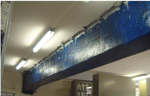
Figure 2-25 Repairing intervention on a r.c. beam using CFRP (Mazzolani) [159] by courtesy of F.M. Mazzolani
