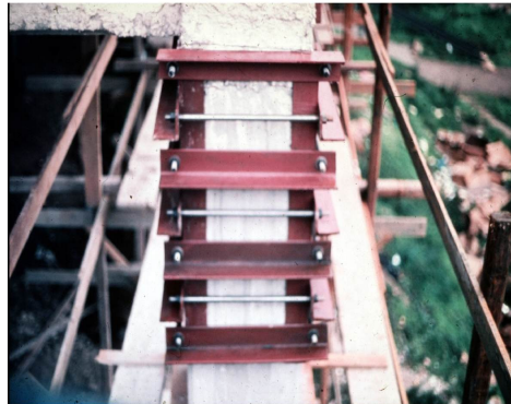
Figure 2-21 Repair of a reinforced concrete column by means of steel angles and ties (Mazzolani) [159]
