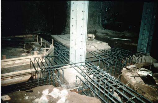
Figure 2-47 Consolidation of an isolated reinforced concrete foundation (Mazzolani) [159] by courtesy of F.M. Mazzolani
