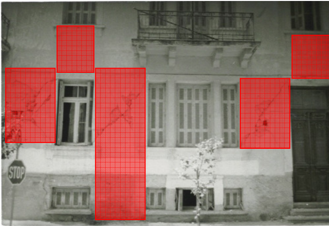
Figure 4-2. Typical damage to a masonry building and possible application of steel/aluminium plates or steel wire mesh for its rehabilitation
