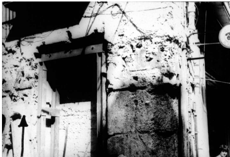
Figure 2-14 Masonry building damaged in time (Mazzolani) [159] by courtesy of F.M. Mazzolani
