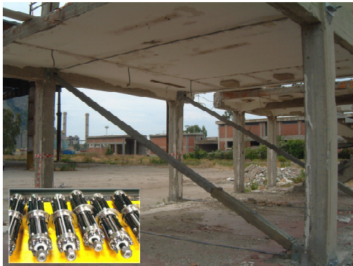
Figure 2-45 Reinforced concrete structure strengthened with SMA braces (Mazzolani) [159] by courtesy of F.M. Mazzolani
