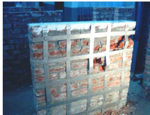
(b) typical failure mode of the walls
