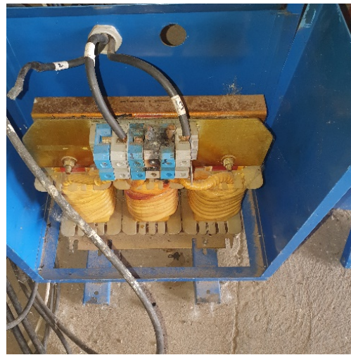
Figure 1.1. b) Dv/Dt filter [19] from a pumping system powered by a photovoltaic generator, that caught fire due to improper use. The DV/Dt filter is used for cables up to 50 m long. For cables longer than 50 m, sinusoidal filters are recommended (picture taken by the author during the visit to a pumping system powered by a photovoltaic generator from Frutas to Rinconada [18]).
