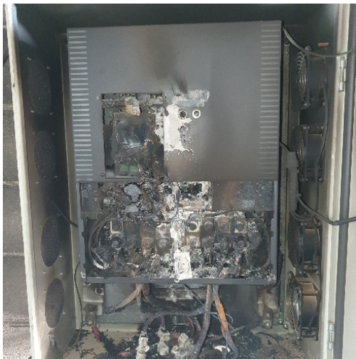
Figure 1.1. a) A variable frequency drive (VFD), from a pumping system powered by a photovoltaic generator, that caught fire due to electric shocks (picture taken by the author during the visit of a pumping system powered by a photovoltaic generator from Frutas to Rinconada [18]).
