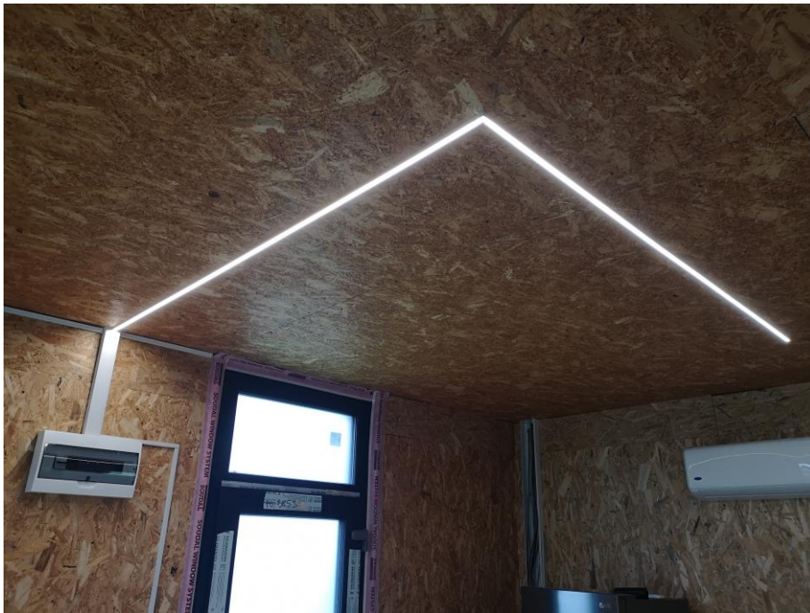
Figure 4.32. Installed lighting system – LED strips
