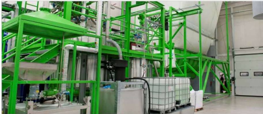
Figure 1.18 The repolyol plant at IKANO, in Poland [49]
