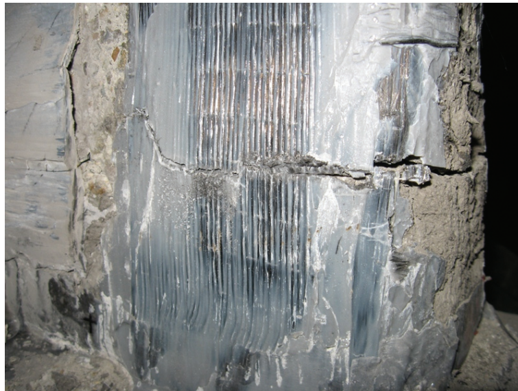
Figure E.120 Failure detail PRCWP 5-S/E3-T/R: the same failure is observed at the opposite face of pier#2 (obs grid 2-2 rear)
