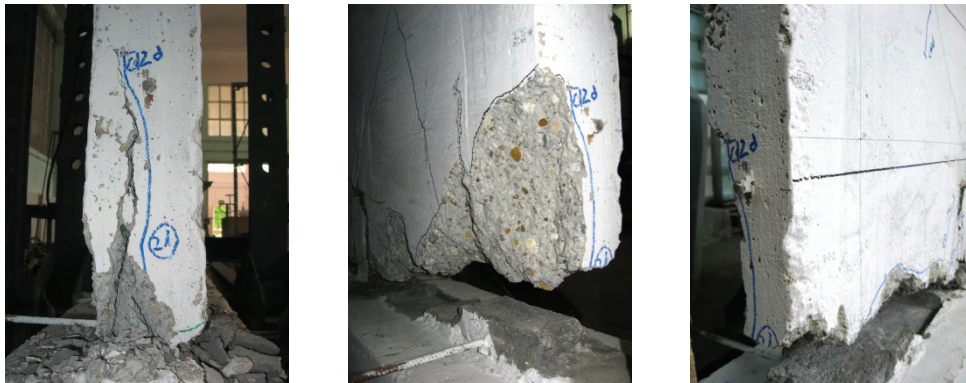
Figure E.30 Failure detail PRCWP 3-S/E1-T: concrete spalling and crushing at the inside toe of pier#2 (obs. grid 3-2)
