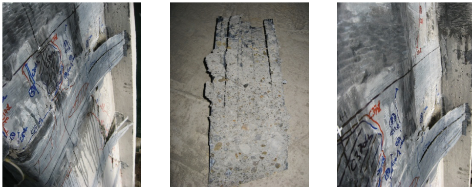
Figure E.117 Failure detail PRCWP 5-S/E3-T/R: FRP strip-end peeling-off at the pier#2-to-wing connection (obs. grid 1-1, 1-2)
