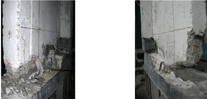
Figure E.51 Failure detail PRCWP 5-S/E3-T: concrete crushing at the inside toe of pier#1 (close-up on grid 3-3)
