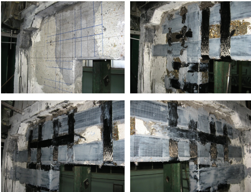
Figure B.7 FRP layout detail at the pier-to-beam connection of PRCWP 5-S/E3-T/R
