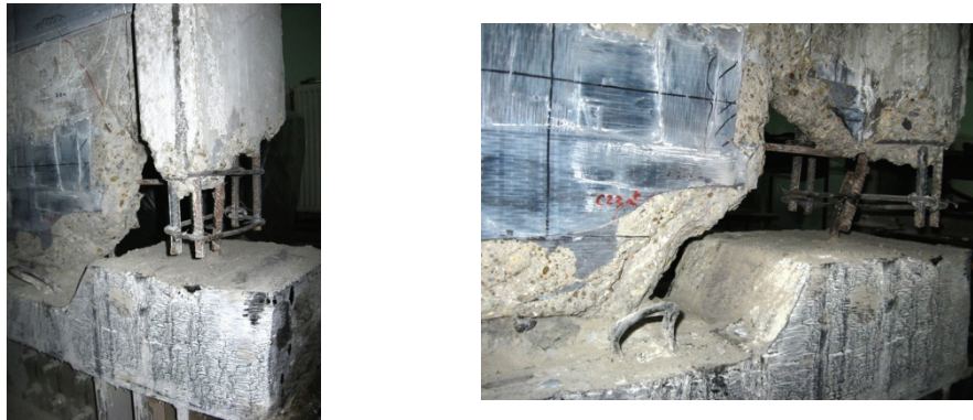
Figure E.90 Failure detail PRCWP 4-S/E1-R/T: the outside toe of pier#2 after removal of the crushed concrete (observation grid 2-2)
