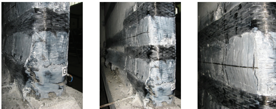
Figure E.71 Failure detail PRCWP 3-S/E1-T/R: bulging of vertical FRP at the toe of pier#2 (observation grid 3-2)
