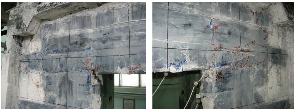
Figure E.145 Failure detail PRCWP 6-S/E3-R/T: FRP bulging and fracture at the spandrel to pier connections (obs. grids 4-4 and 1-1)
