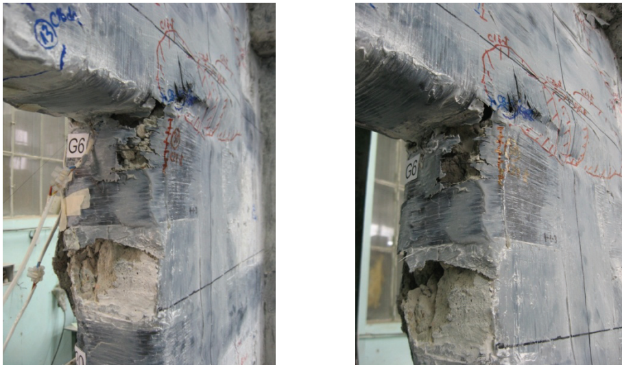
Figure E.144 Failure detail PRCWP 6-S/E3-R/T: FRP confinement fracture at the spandrel-to-pier#2 connection (obs. grid 1-1)
