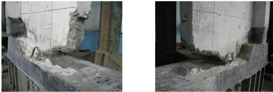
Figure E.52 Failure detail PRCWP 5-S/E3-T: the pier toes after crushed concrete was removed (close-up on observation grid 3-3 and 2-2)
