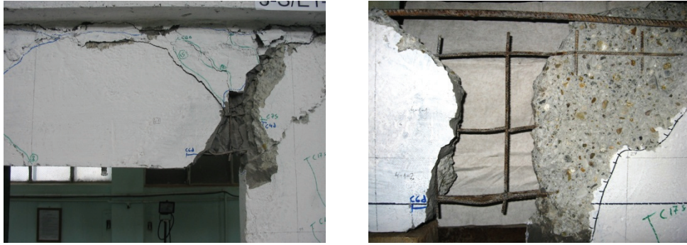
Figure E.32 Failure detail PRCWP 3-S/E1-T: concrete crushing at the spandrel-to pier#2 connection (close-up on grid 4-1)
