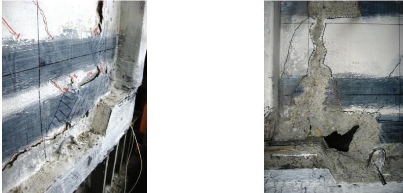
Figure E.72 Failure detail PRCWP 3-S/E1-T/R: FRP debonding and concrete crushing at the outside toe of pier#2 (observation grid 2-2)
