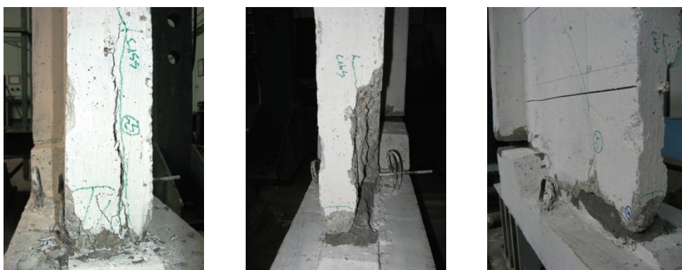
Figure E.31 Failure detail PRCWP 3-S/E1-T: concrete spalling and crushing at the inside toe of pier#1 (obs. grid 3-3)
