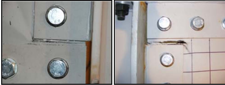
Figure 21 - Infill plate corner tearing
