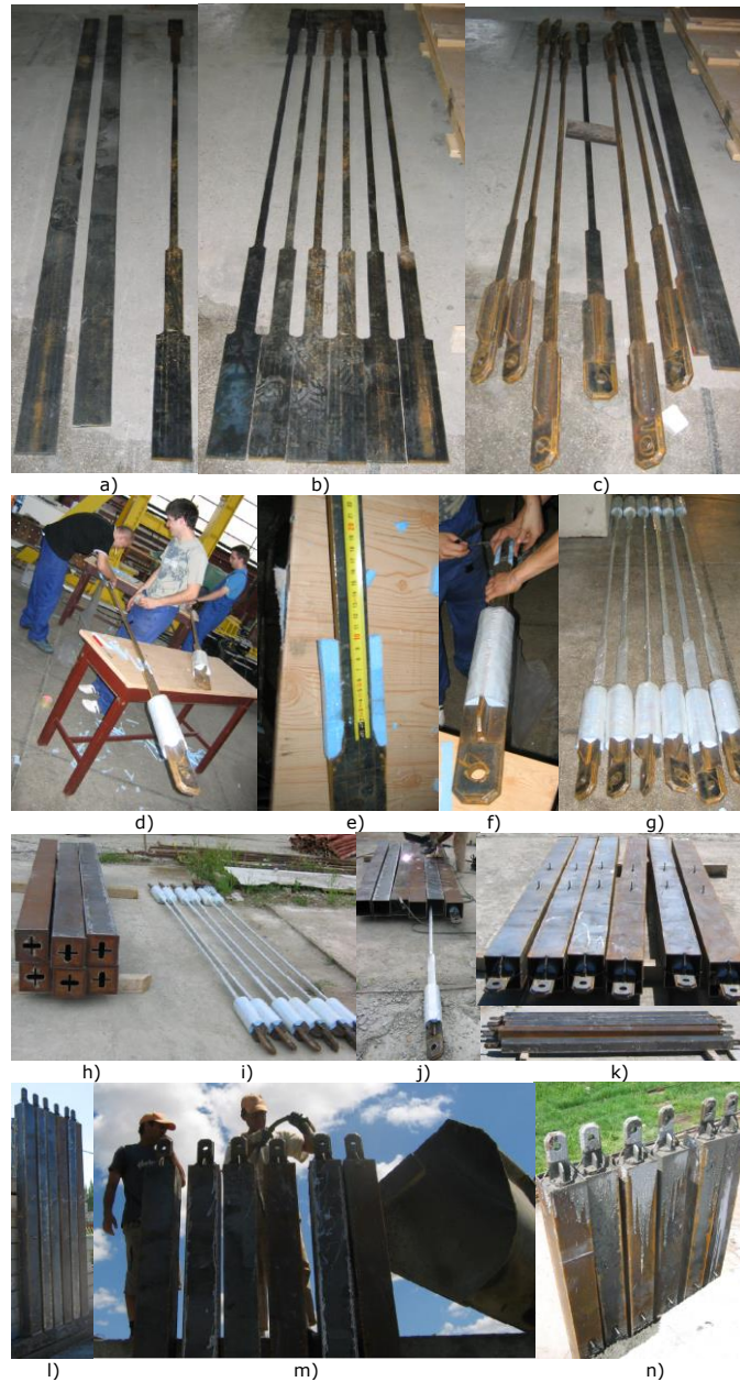
Steps were followed in order to built BRB elements a) and b) mechanical cut; c) welding of the web stiffeners; d) and e) positioning of polystyrene (to permit longitudinal deformations); f) and g) wrapping of the unbonding material (PVC transparent film of 1mm thickness); h), i), j) and k) insertion and calibration of the wrapped steel core into restraining steel tube; l) vertical positioning of the BRB element; m) infill of the restraint material (concrete).
