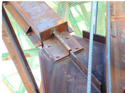
Figure 2.68 Connection detail for application of BRB to Constructions of the Tzu-Chi Culture Building ( TV Station ) [43]
