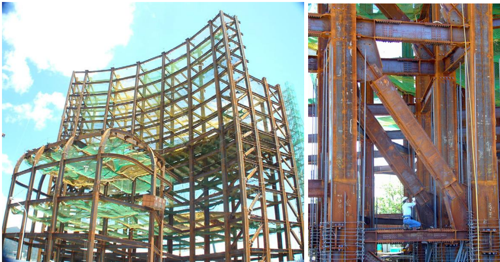
Figure 2.67 Application of BRB to Constructions of the Tzu-Chi Culture Building ( TV Station ) [43]
