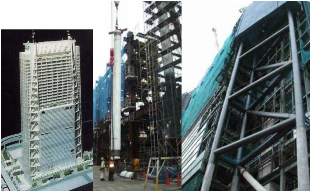
Figure 2.58 Nippon TV Headquarters, Tokyo (1.4 million s.f., 32+2 storeys, h=630 ft, 68 braces, L=60 ft., P_y = 2400 kips) [26]
