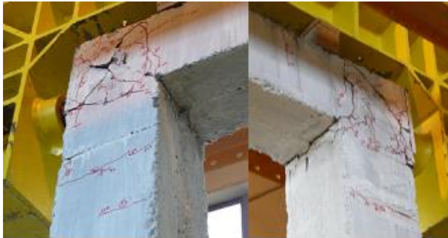
Figure 6.27 RC frame under cyclic load – failure of the node
