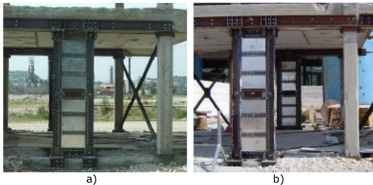
Figure 2.32 Global view of the structure retrofitted by means of: a) steel shear panels; b) aluminum shear panels [10]
