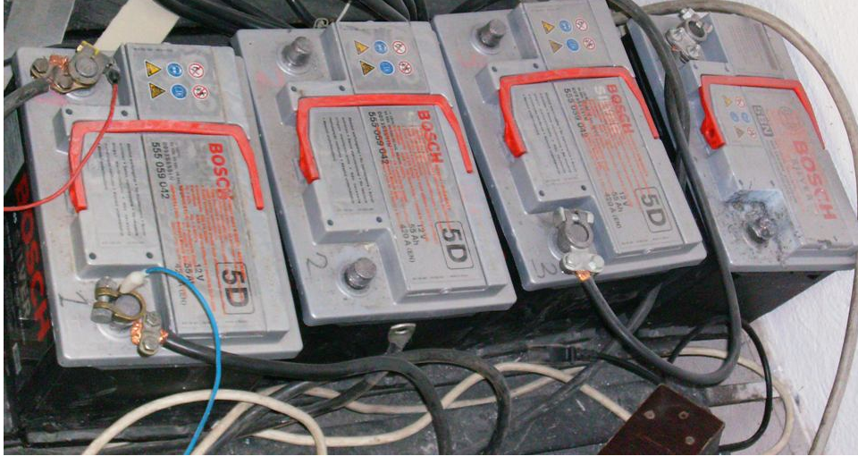
Fig. 7.3. 4x12V valve regulated lead acid batteries
