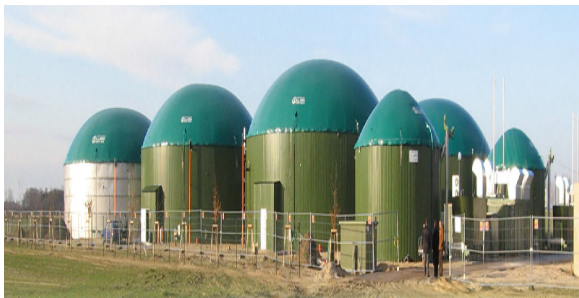
Photo 1. Digesters for anaerobic fermentation
