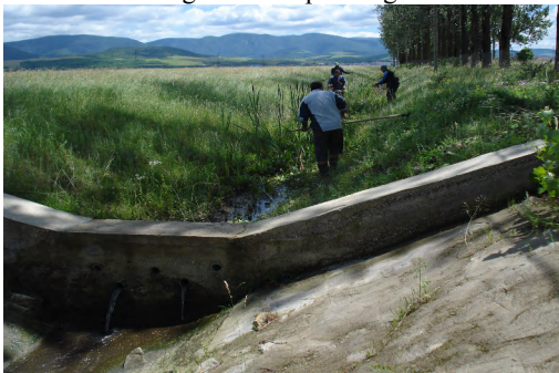
Photo 3 – Main drainage channel CP41 threshold drop of concrete, works for the destruction of aquatic vegetation and grassy (2010)
