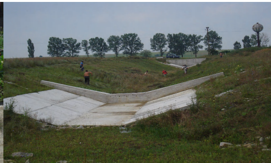
Photo 4 -Main drainage channel CP41 threshold drop of concrete, works for the destruction of aquatic vegetation and grassy (2010)
