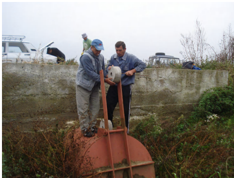
Photo 7 – Under-crossing the dike with metallic dampers Channel CCS42 Lisava Valley Maintenance and repairs works to the metallic damper counterweight (2010)
