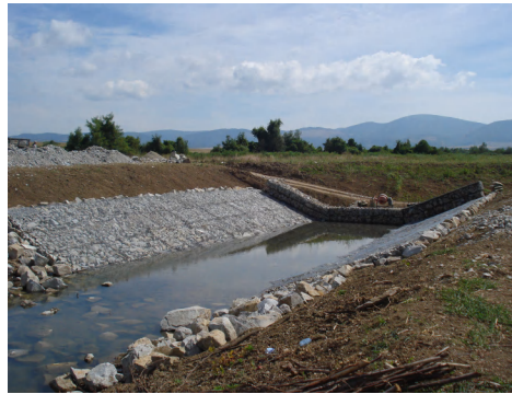
Photo 22 – Drop from gabions with rough stone on Lisava Valley at km 5+300 (2008)
