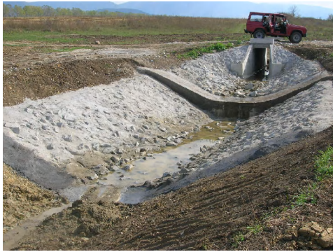
Photo 15 – Pipe DN1200 (of caissons) and drop of concrete and rough stone on drainage channel CS403 (2008)
