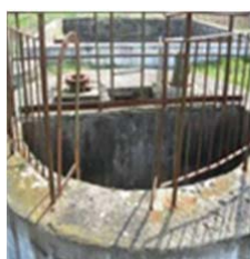
Sludge pumping station
