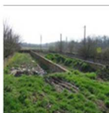
Sludge drying platform
