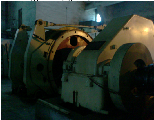
Figure 5 – Example of machines from Lupeni mine
