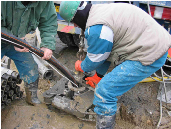
Fig. 9. Real installation of VRT485 bus of sensor
