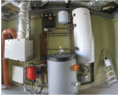
e) Technical room
