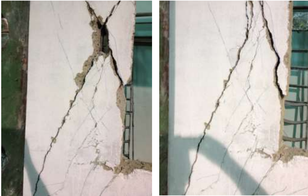
Figure 4-2 – Failure details of PRCWP 15
