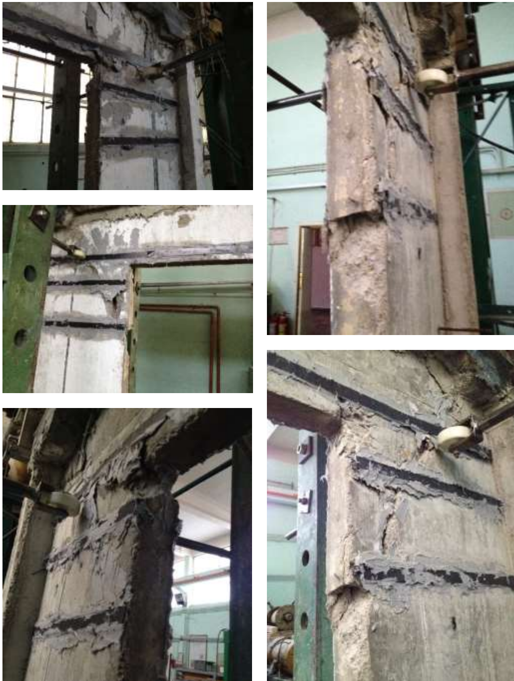
Figure 4-9 – Failure details of PRCWP 18-L3-E3-TR
