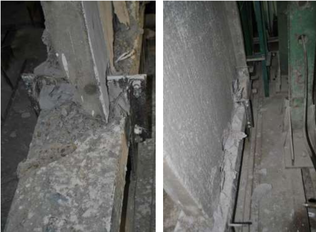
Figure 4-3 – Failure details of PRCWP 16-L1-E1-T
