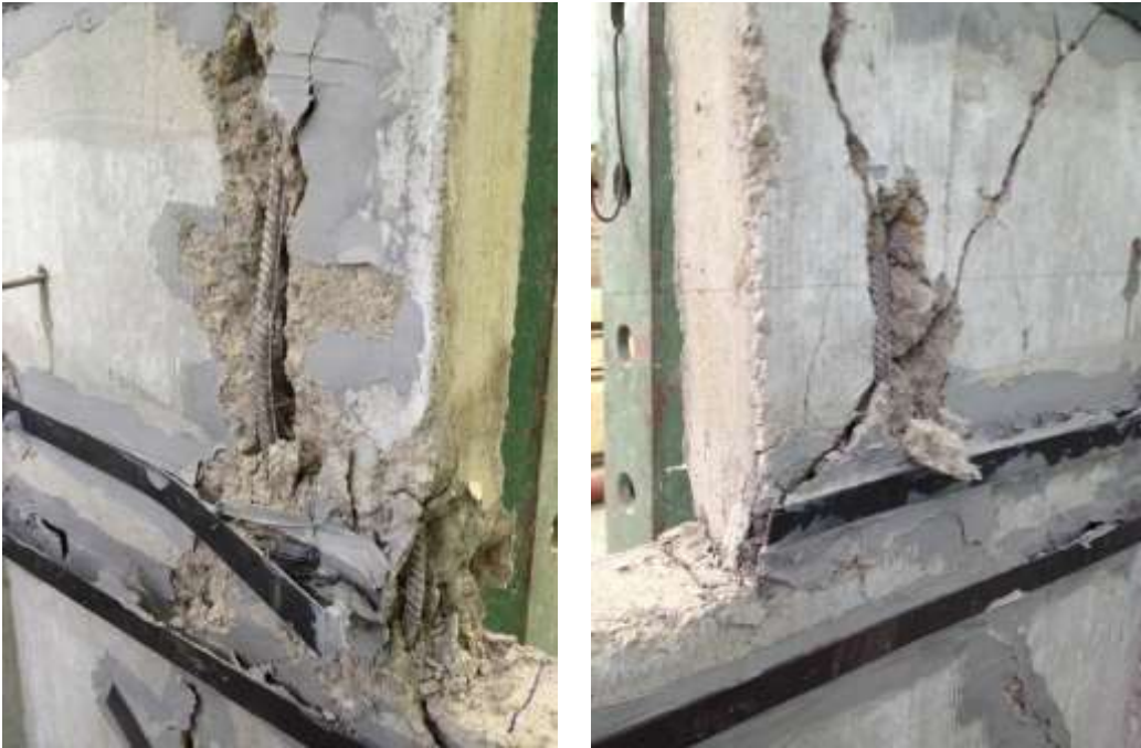
Figure 4-8 – Failure details of PRCWP 17-L3-TR
