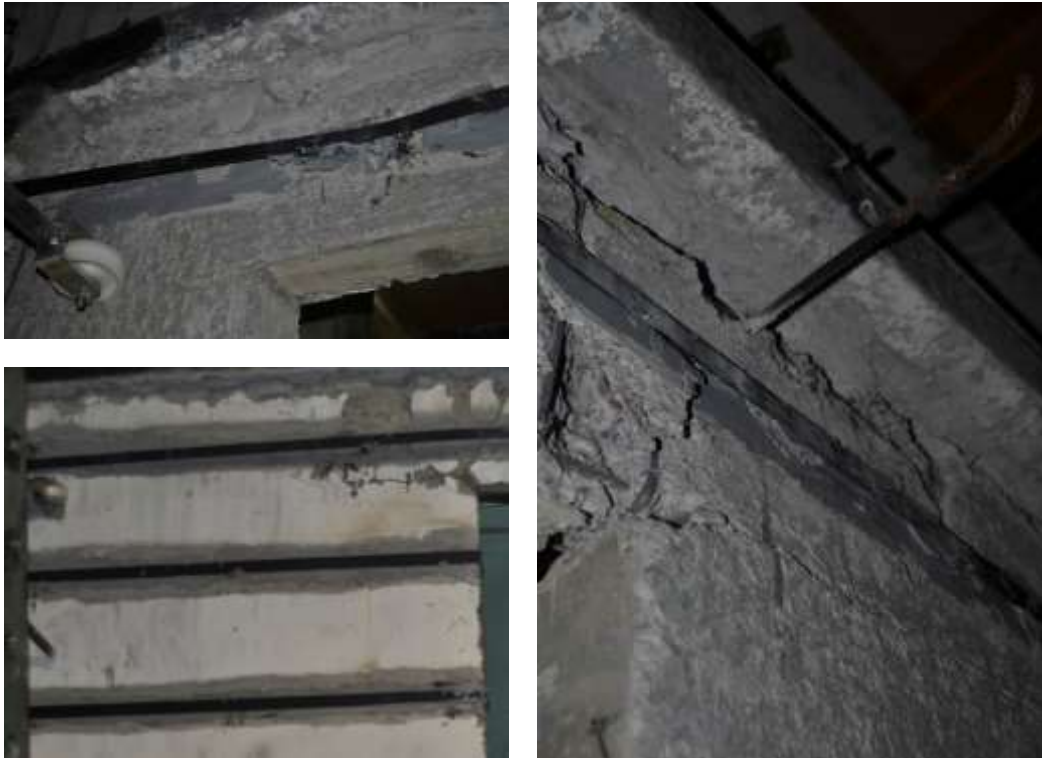
Figure 4-7 – Failure details of PRCWP 16-L1-E1-TR
