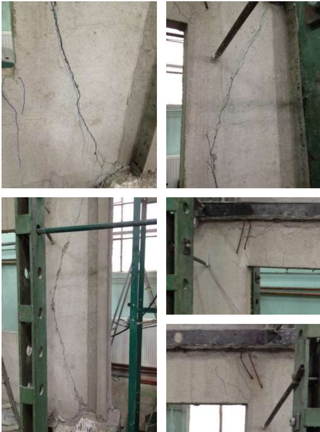
Figure 4-4 – Failure details of PRCWP 17-L3-T
