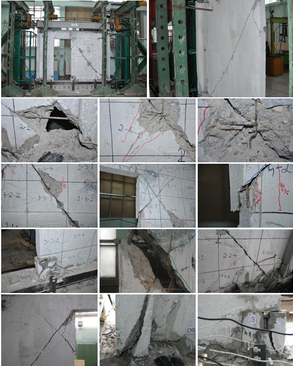
Figure 2.21 – PRCWP (7-E1-T) failure details [108-110, 112, 115]
