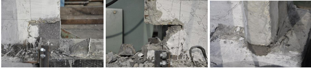
Figure 2.22 – PRCWP (8-E3-T) failure details [108-109, 112, 115]
