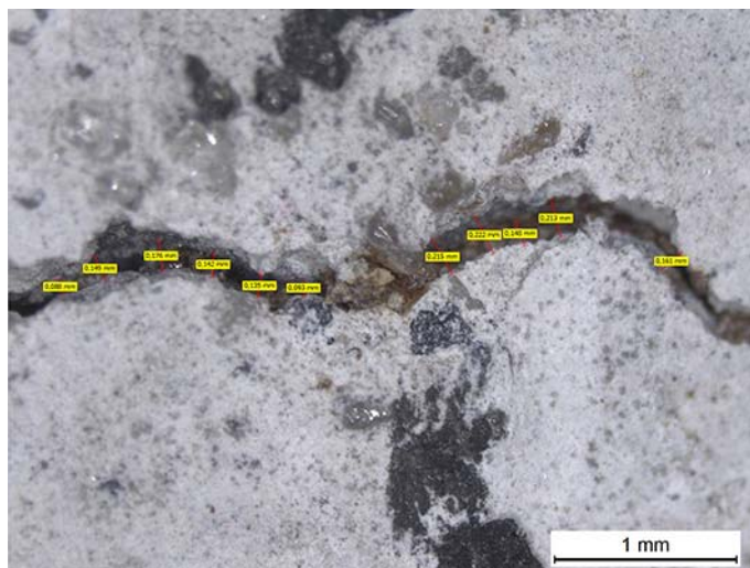
Figure 3.8. Tortuous profile of the crack
