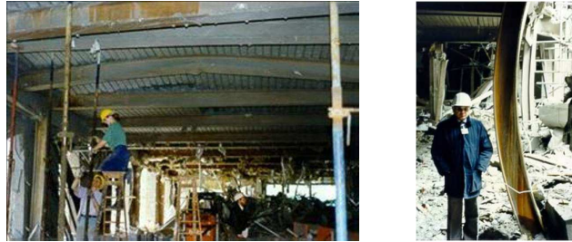
a) damage to composite floors b) ground floor steel columns Figure 2.2 Exchequer Court bombing, St Mary's Axe, London 1992 [14]
