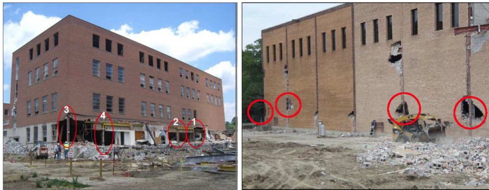
a) Ohio Union building, 2007 b) Bankers Life and Casualty Company, 2008 Figure 2.26 Buildings with exposed columns to be sequentially removed before testing [88]
