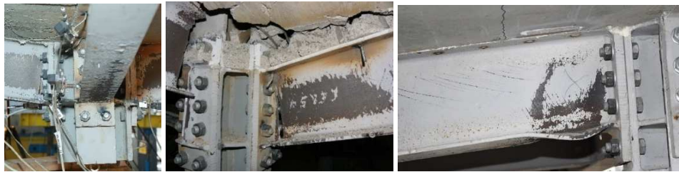
a) fracture at beam B2-B3 b) complete beam fracture c) Column B1 connection at point B Figure 3.73. Detailed views of the connection [153]
