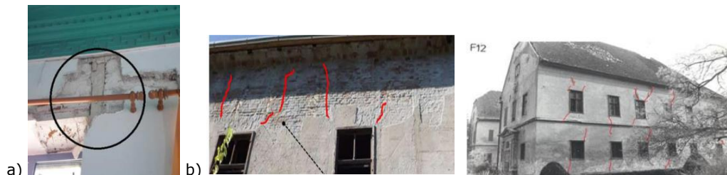
Figure 3.44. Vertical cracking in-plane failure mechanism observed at masonry buildings in the epicentre of : a) Plomari [197]; b) Banloc earthquake, 1991 [174]
