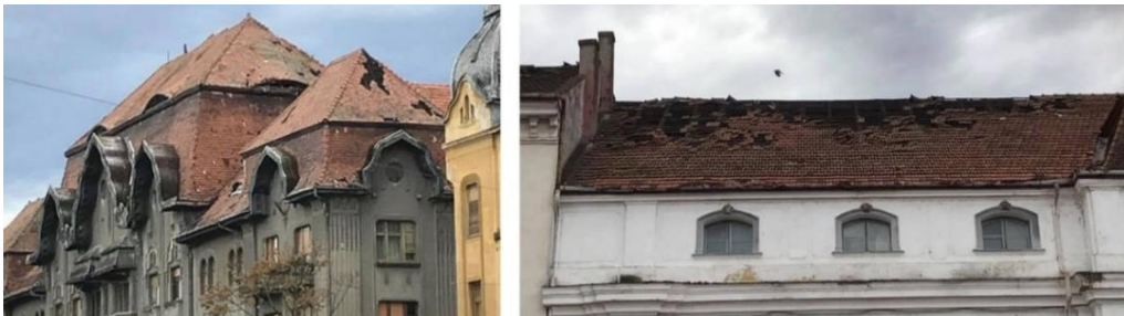
Fig. 2.39. Damage to heritage buildings - wind storm from the 17th of September 2017 in Timisoara (wind velocities of 145 m/s)
