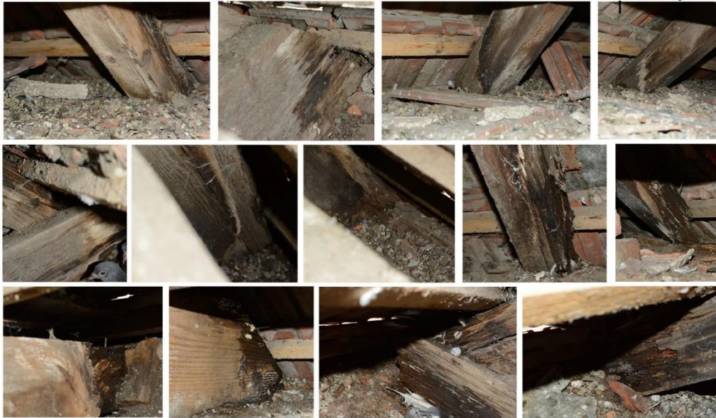
Fig. 2.34 Decay of the timber elements caused by water infiltration
