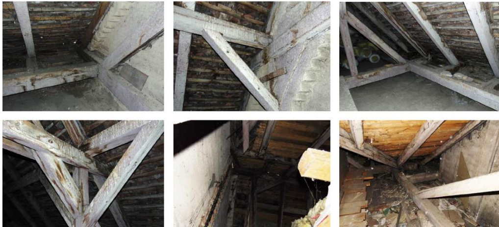
Fig. 5.18 "Victoria" Hotel – decay of the timber roof structure
