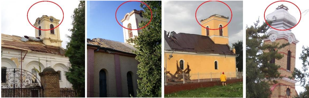
Fig. 2.40 Failure of bell tower roof structures - wind storm from the 17th of September 2017 in Timisoara (wind velocities of 145 m/s)
