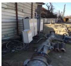
Figure 9. Small panel with alarm system and two secondary electrical panels
