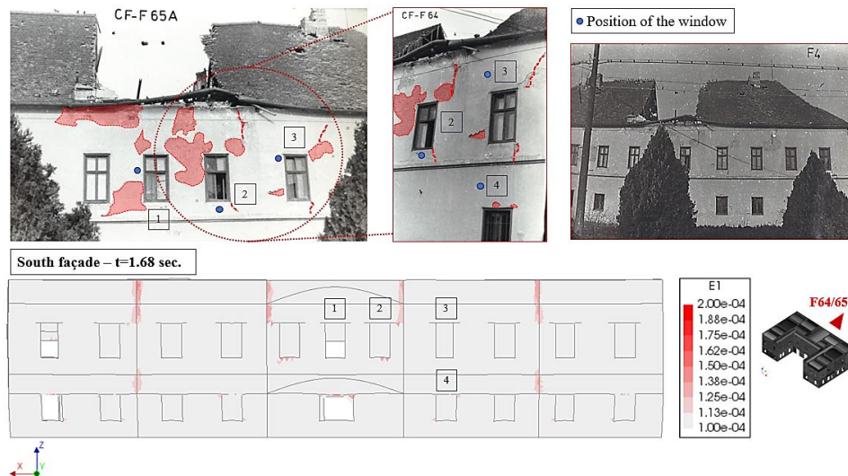
Figure 4.60: Damage correlation depicted in the South façade of the case study building.
