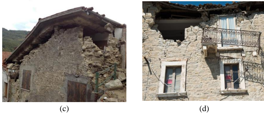
Figure 2.32: Damage identification in Pescara del Tronto [137].
