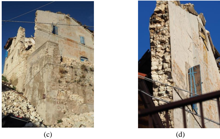
Figure 2.34: Damage observed in Castelluccio di Norcia [137].
