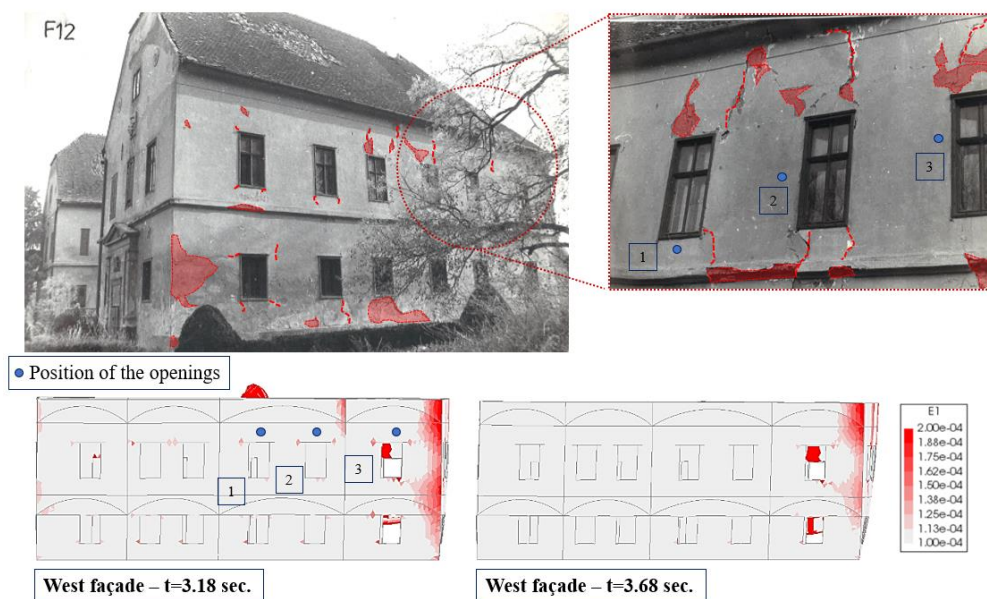
Figure 4.68: Damage deduced near the right corner of the West façade.
