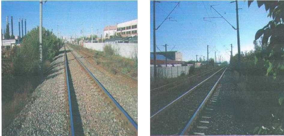
Fig.5.29 Terasament instabil km.628+350 - km.628+600
