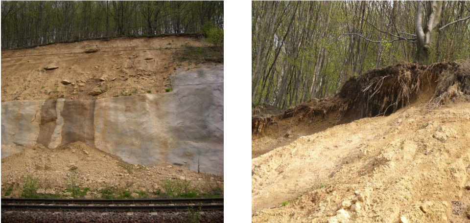
Fig.5.46 Versant instabil linia 116 Simeria - Livezeni km.73+960 - km.74+283
