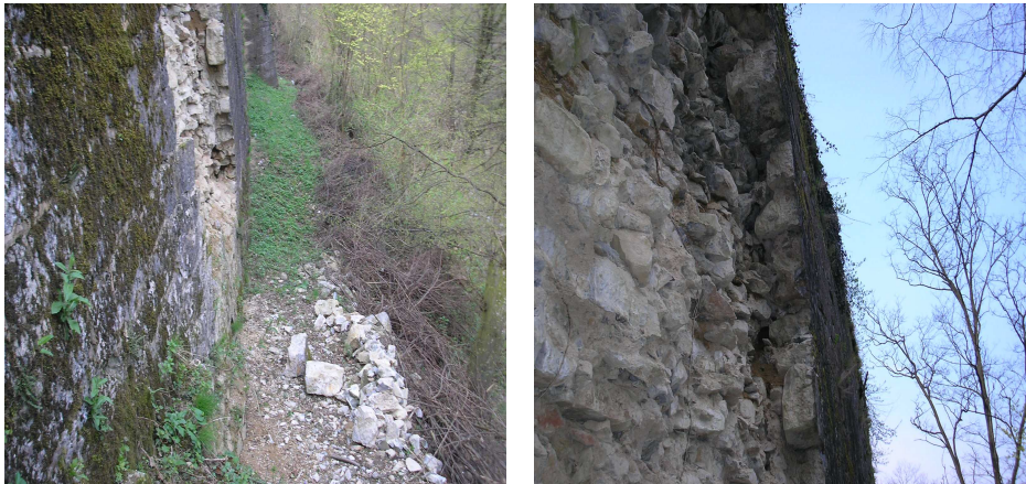
Fig.5.58 Zid de sprijin distrus linia 131 Oravița - Anina km.9+050 - km.9+200
