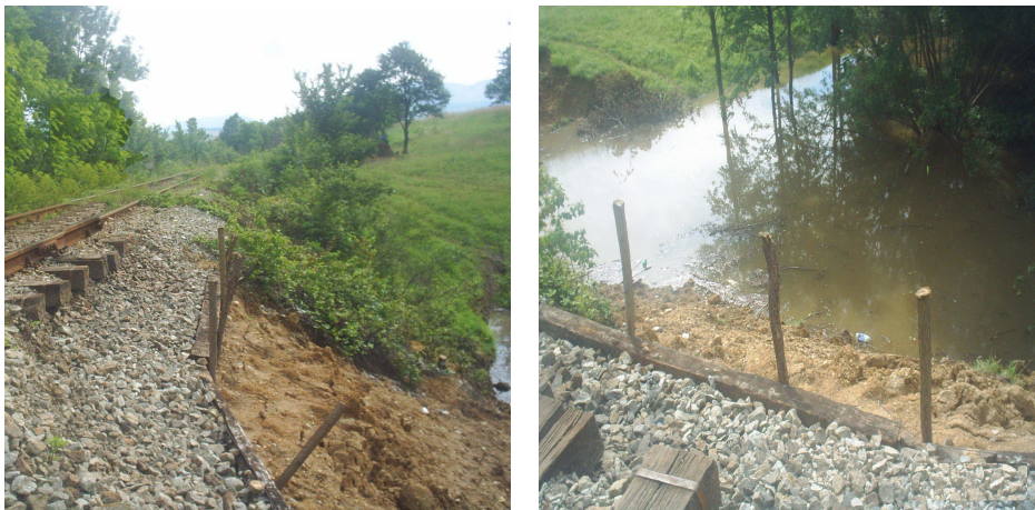
Fig.5.54 Alunecare taluz linia 130 Berzovia - Oravița km.54+475 - km.54+525
