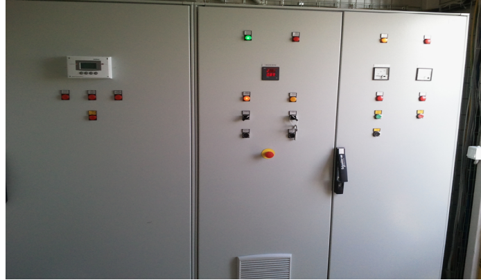
Fig.5.2. Energy conversion and storage equipment.
