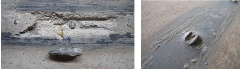
Fig. 5-36. Detail of concrete and connector after cyclic loading
