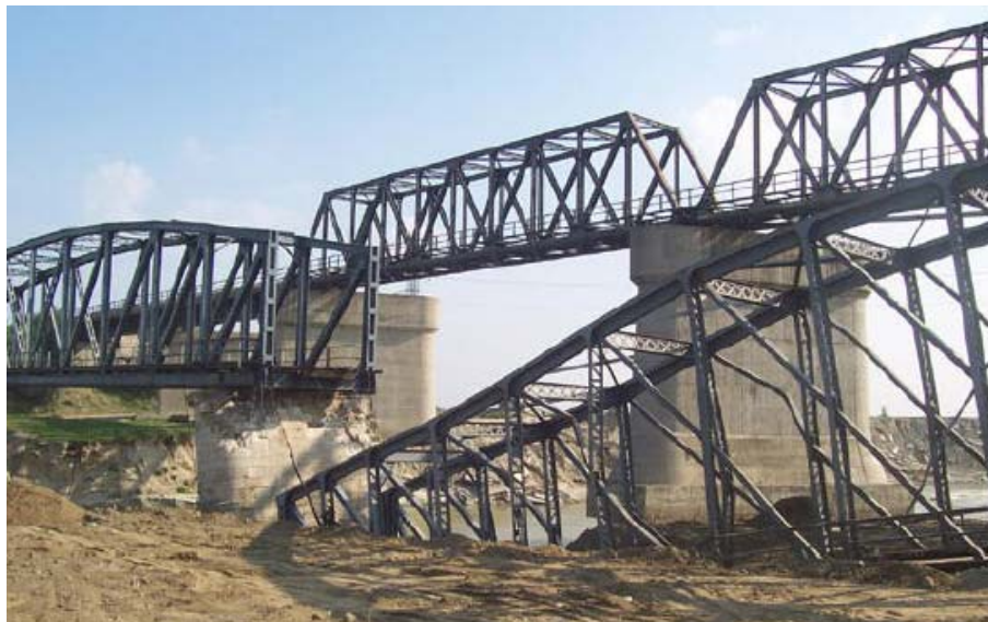
Figure 2.2 – Collapsed railway bridge near Giurgiu, Romania (Floods, 2008)
