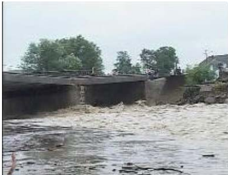
Figure 2.1 – Collapsed bridge in Marginea, Suceava County, Romania (Floods, July 2008)
