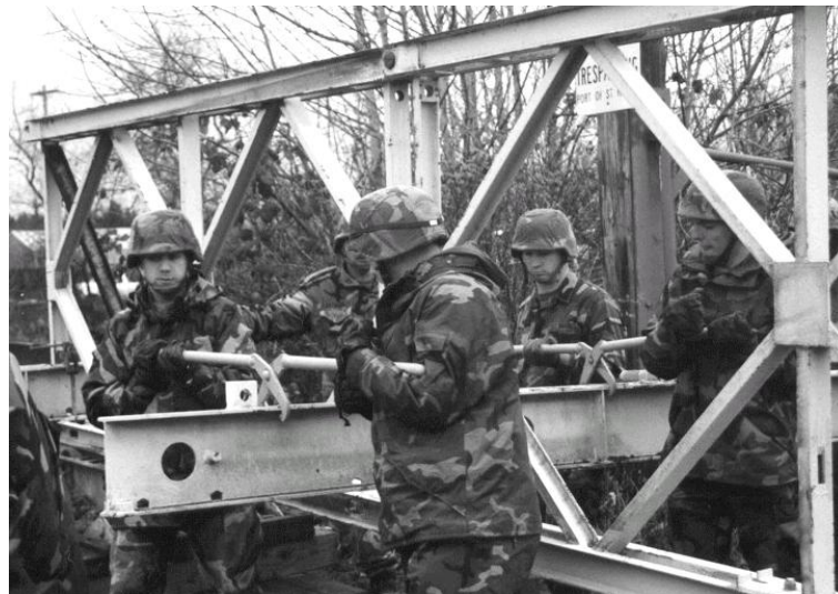
Figure 3.20 – Assembly of a Bailey Bridge [24] (Image courtesy of the Oregon Military Department, US )
