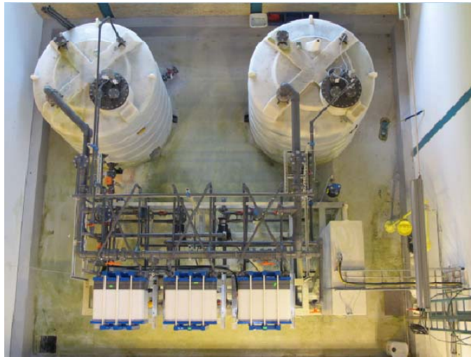
Fig. 2.23. Vanadium battery installation seen from above: electrolyte tanks in the back, 3 cell stacks at the front.
