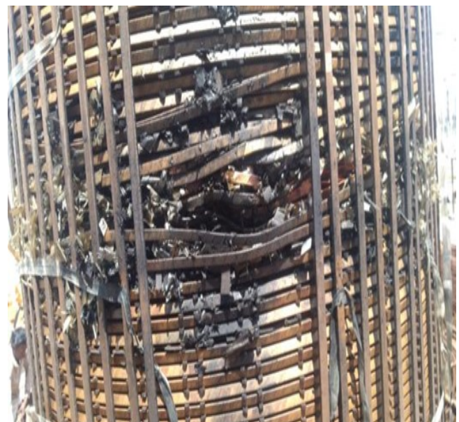
Fig. 15. Buckled tertiary winding with turn to turn short
