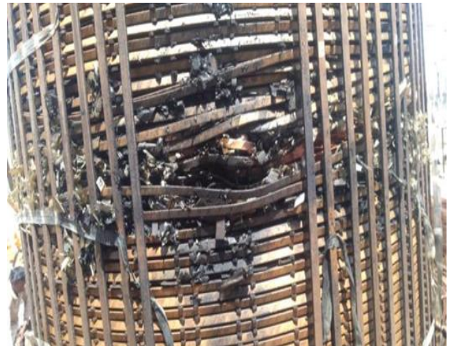
Fig. 14. Buckled tertiary winding with turn to turn short
