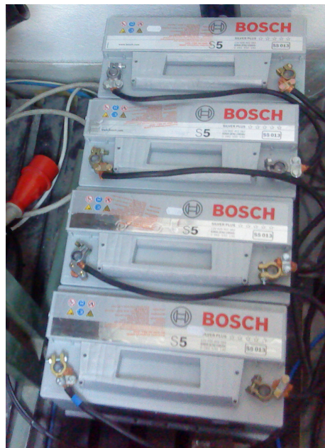
Figure 6.3. Series connected lead-acid Bosch automotive batteries
