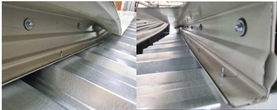
Figure 3.63 Detail of the failure zone of the liner tray: interaction between local+distortional buckling of the wide flange and web crippling
