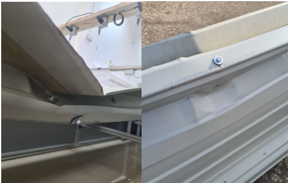
Figure 3.59 Detail of the failure zone of the liner tray: interaction between local+distortional buckling of the web and local buckling of the wide flange
