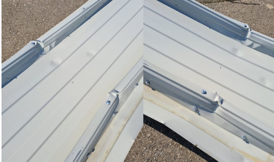
Figure 3.43 Detail of the failure zone of the liner tray: interaction between local+distortional buckling of the narrow flange and local+distortional buckling of the webs
