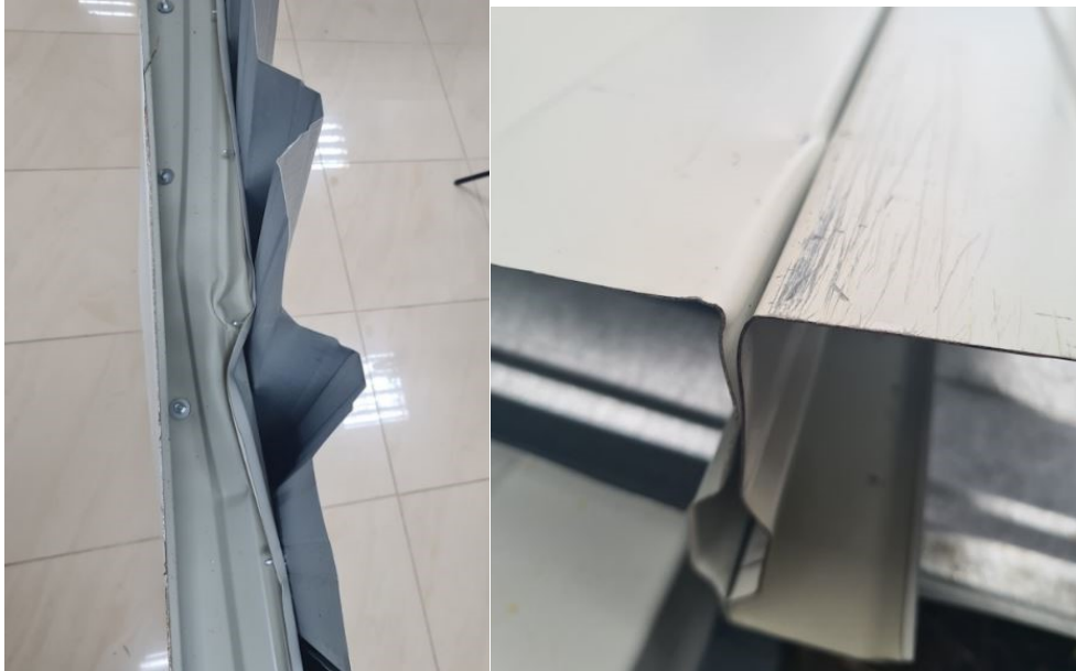
Figure 3.47 Detail of the failure zone of the liner tray: web crippling (left) and wide flange local buckling in the support area (right)
