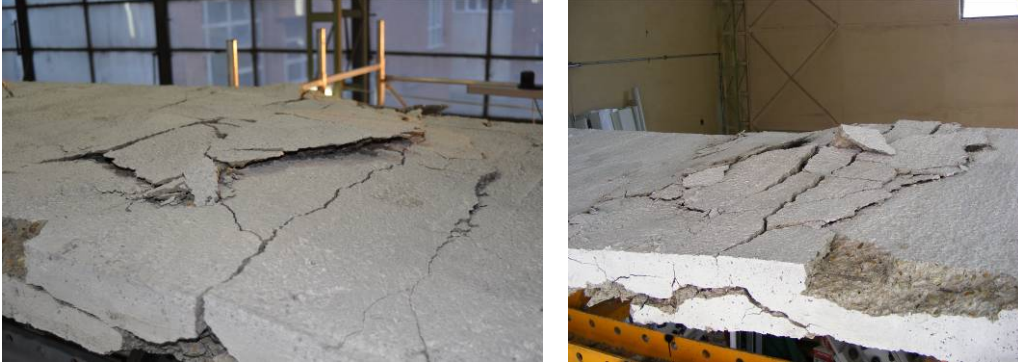
Fig. 3.49. Damage of the concrete slab during the tests of EBF_Comp_LD1 and LD2
