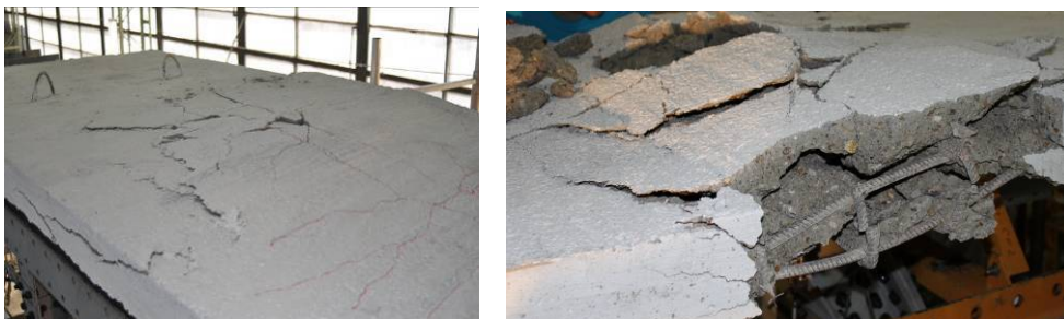
Fig. 3.45. Damage of the concrete slab during the tests of EBF_LF_Comp1 and Comp2
