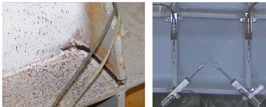
Fig. 3.66. Failure of the welds in the beam-column joint and CWP distortion
