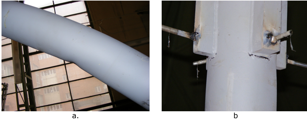
Fig. 3.30. a) Plastic hinge formation at the middle of the CHS brace; b) Crack development near the connection of the CHS brace with the pinned base plates
