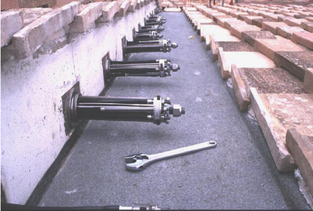
Fig. 2.31. SMA devices installed on the roof of Basilica S.Francesco in Assisi [23]
