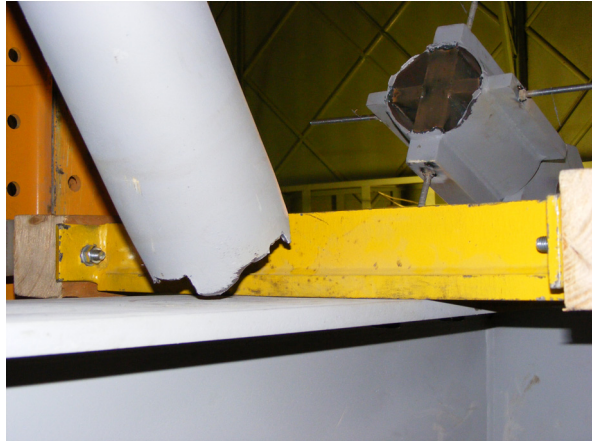
Fig. 3.25. Failure of the connection between the CHS brace specimen and connection plates of the pinned support
