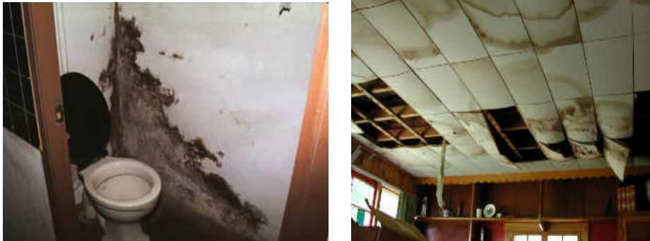
Fig. 5.67. Effects of excessive humidity
